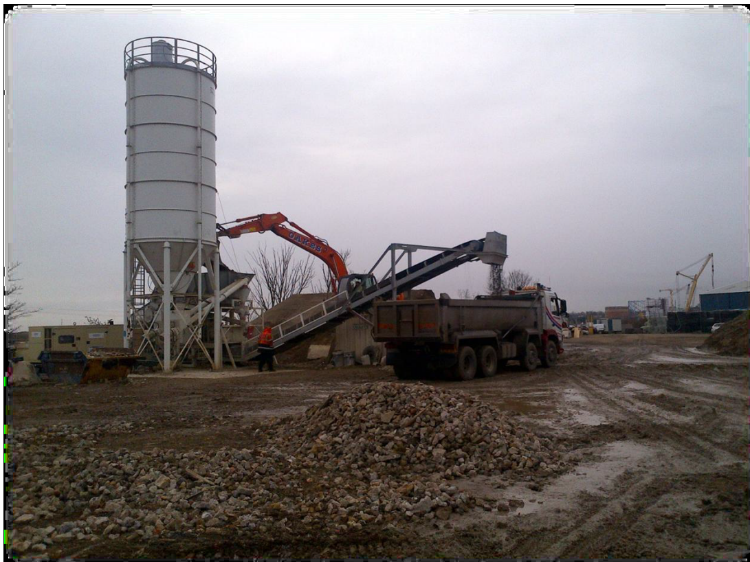
Figure 1: Typical Looking HBM Plant
